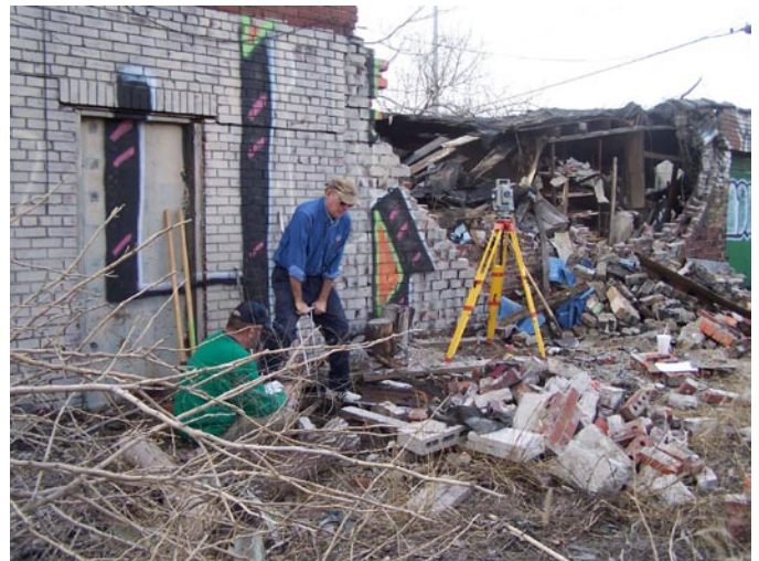
John Kelly collecting a core sampling prior to demolition of the hardware store built atop a newly acquired mound site in East St. Louis. See page 6 for more photos of this site.
